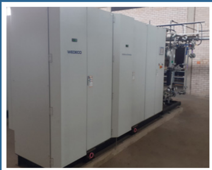
Figure 3: Electrical and Control System for the Ozone Generator
