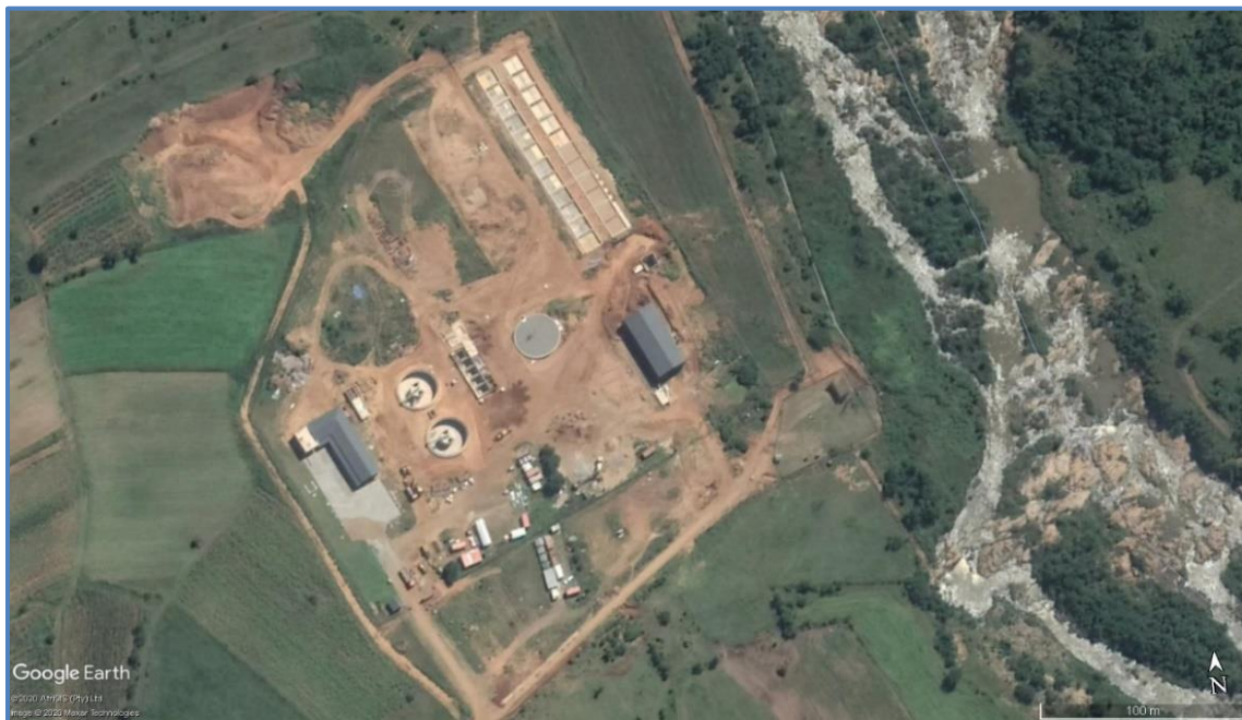
Figure 17.75 Construction of new 15 Mℓ /day WTP at Frischgewaagd along the Phongola River
