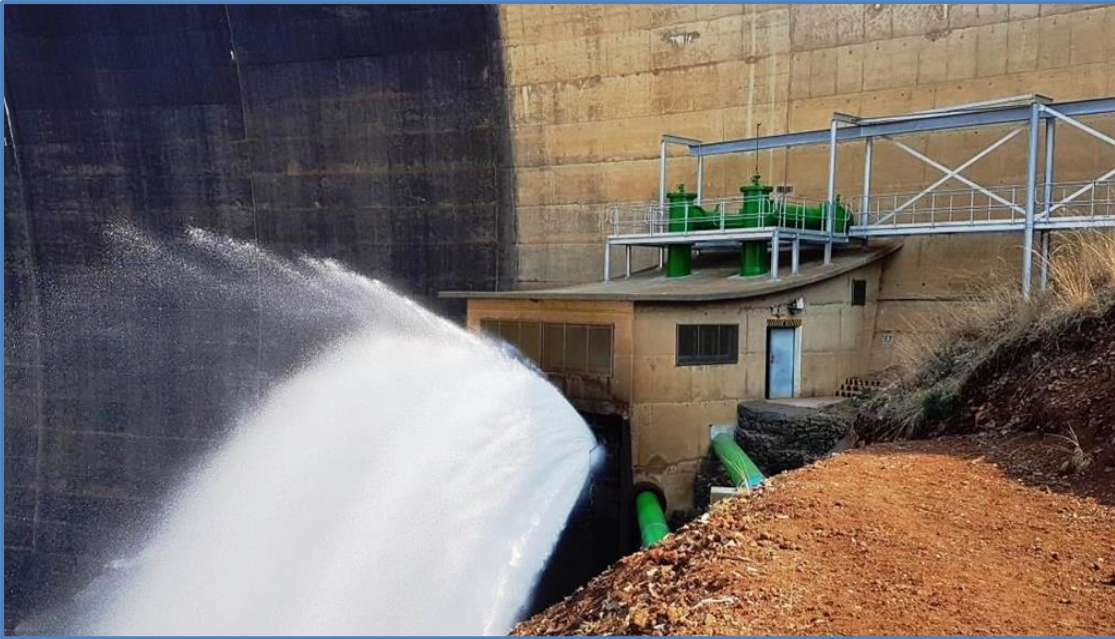
Figure 12.47 Abstraction point (Craigie Burn Dam)
