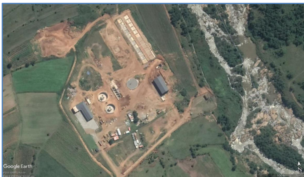
Figure 17.75 Construction of new 15 Mℓ /day WTP at Frischgewaagd along the Phongola River (Google Earth 2020: website).
